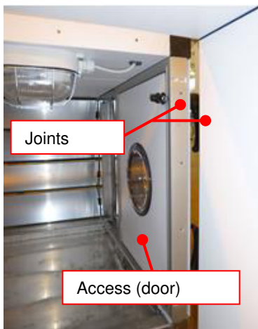
Figure 36: AHU separation accessible via door
