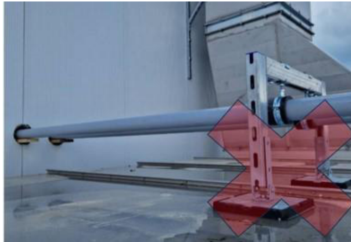
Figure 15: Improper on-site piping
