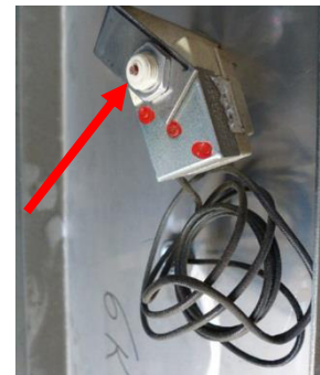
Figure 77: Thermostat with uncovered reset button
