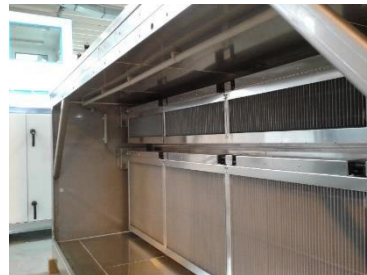
Figure 169: Electrostatic filters in the filter frame
