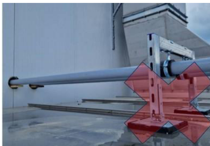
Figure 38: Improper on-site piping
