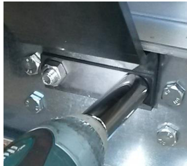
Figure 30: Fixing of the metal sheet and the monobloc crane lifting lug with nuts
