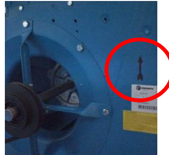
Figure 207: Rotation marking of housing fans
